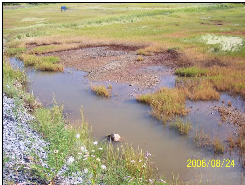
Figure 8. Bridge and culvert replacement project resulting in marsh ponding and dying vegetation. BOAT MEADOW, EASTHAM
