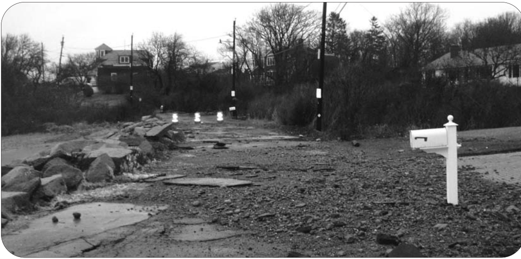
In addition to being costly to repair, roads damaged by storms can become hazards for rescue personnel and others. This road in Rockport, Massachusetts, was destroyed by a 2007 nor'easter.
