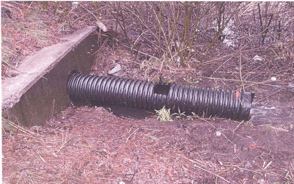
Figure 3-3: Flow structure at the Cherry Hill site for high flow conditions. The existing drainage pipe at the site was “extended” with a ribbed pipe. Walls within the pipe extension were smooth (i.e., not ribbed). Flow was measured by placing the Global Water flow probe into the center hole, that was cut into the pipe extension.
