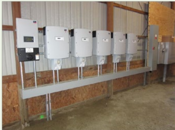
The five (5) central inverters located in the maintenance building convert the panels' direct current (DC) to alternating current (AC) and are of the correct electrical quality and characteristics for on-site use and export to TLMP.
