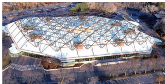
The 158,000-square-foot roofing system at the Carver-Hawkeye Arena at the University of Iowa features membrane Sika Sarnafil recycled from the old roof, which had been damaged by a severe storm.
