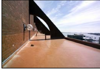
Above: The new roof at the Marriott Long Wharf Hotel in Boston
