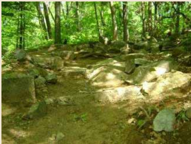
Erosion on the Skyline Trail
