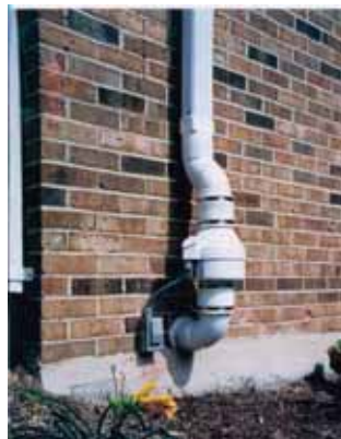
Figure 4-3: Outside Fan and Piping
