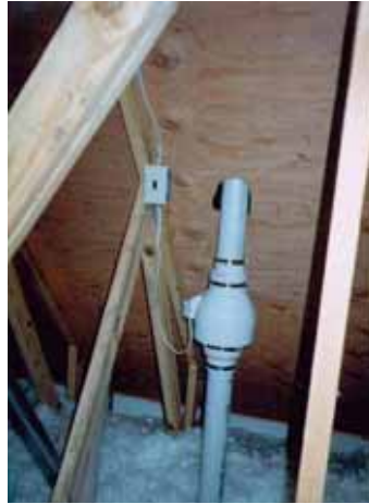
Figure 4-4: Fan in Attic
