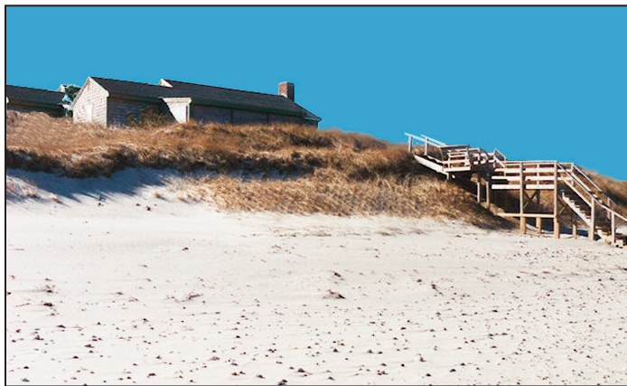
The photo on the left shows a dune nourishment project where sand was added in front of the eroded face of an existing dune. The sand was planted with beach grass to enhance the protection provided to the house behind it.
