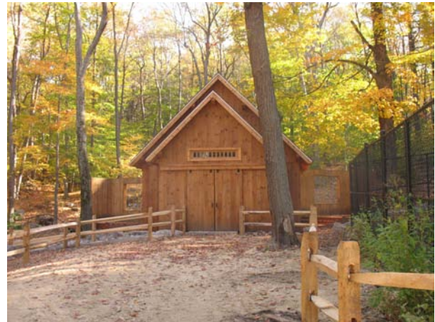
New Rocky Outcrop exhibit enclosure and accessible path, under construction, Fall 2008 (Pressley Associates).
