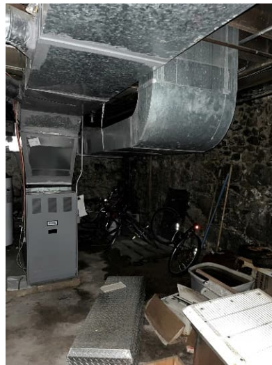
Figure 8: Large duct that reduces basement headroom
