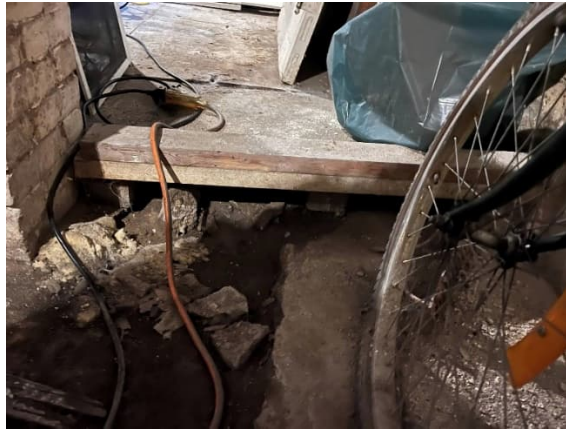
Figure 7: Non-level walking surface in basement
