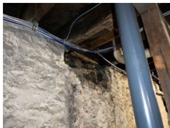
Missing Stone at Foundation Wall
