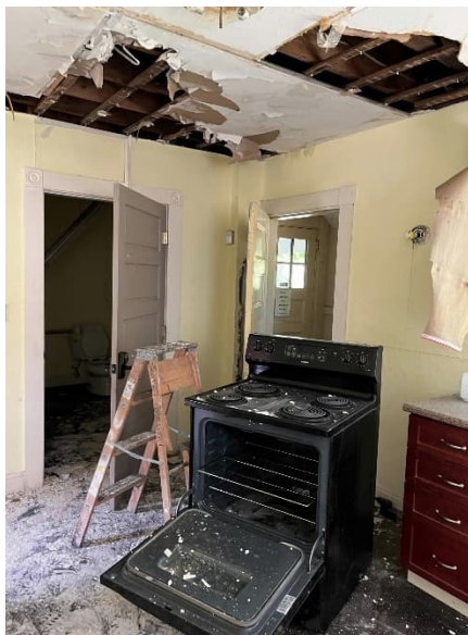
Figure 7: Floor/ceiling assemblies in disrepair
