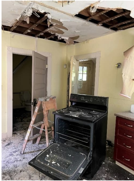
Figure 5: Floor/ceiling assemblies in disrepair
