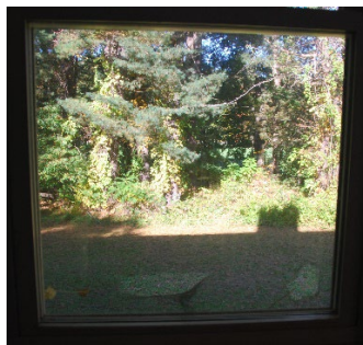
Damaged Screen & Damaged Glass
