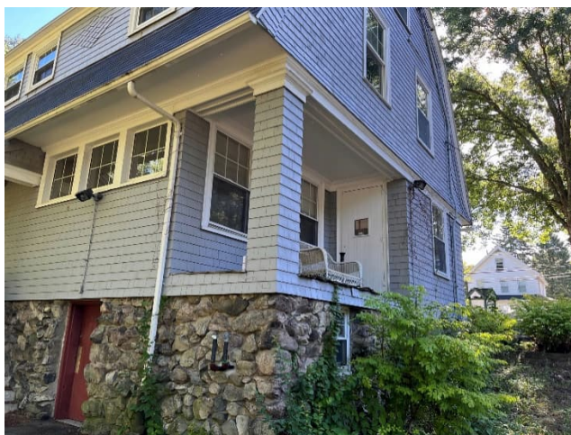
Figure 3: Lack of guards at basement, rear stair, and exterior porch
