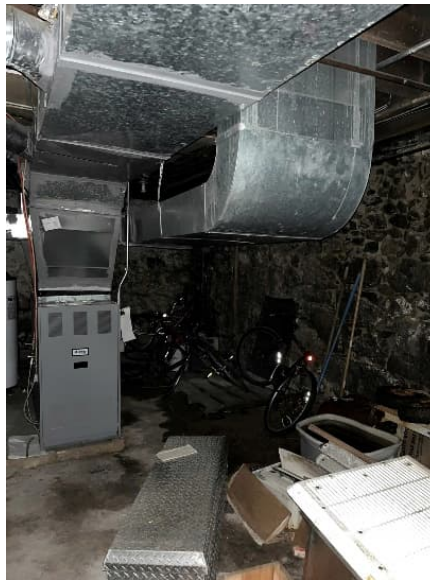
Figure 12: Large duct that reduces basement headroom
