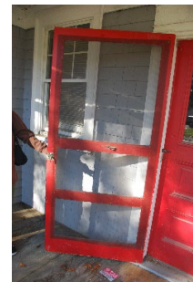
Screen at Front Door
