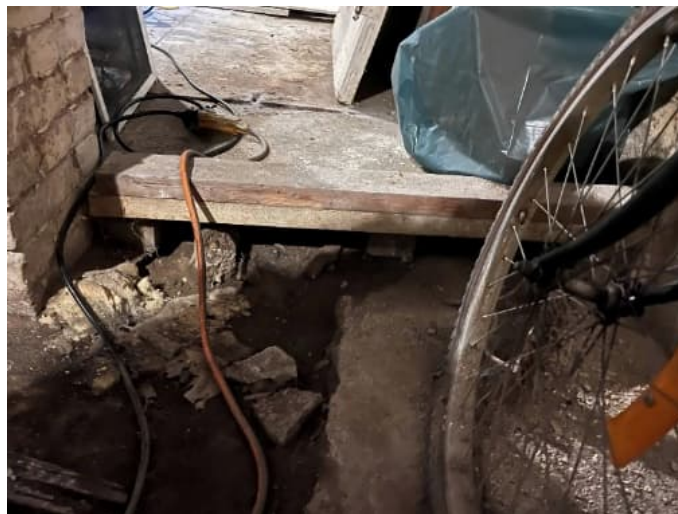
Figure 11: Non-level walking surface in basement
