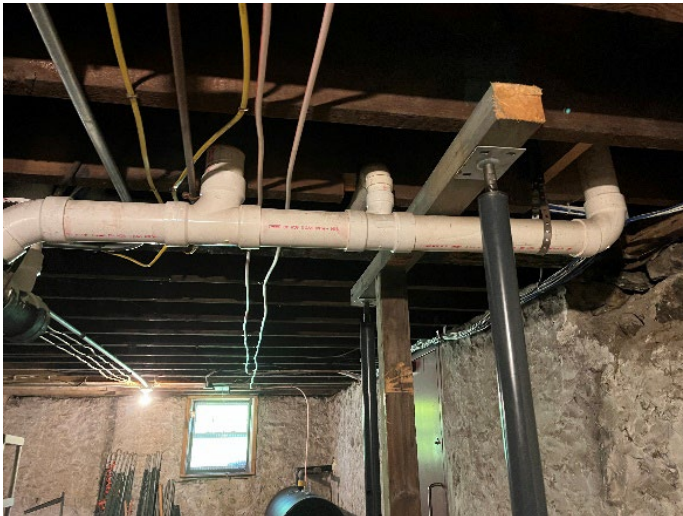
PVC Waste Piping
