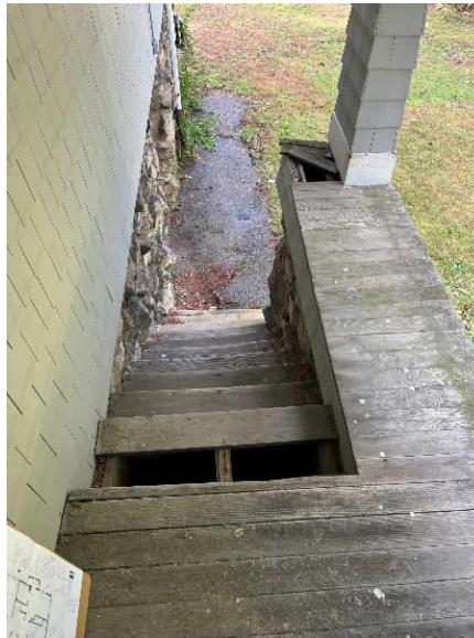
Figure 6: Missing treads and decking at rear stair
