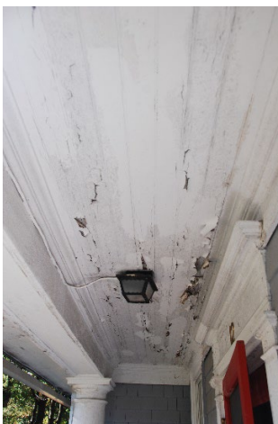
Peeling Paint ant entry soffit
