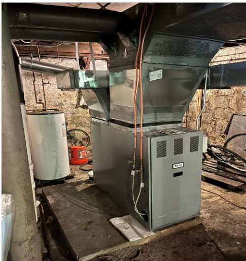
Oil Fired Furnace
