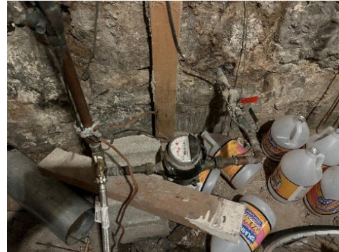
Water Meter and PRV
