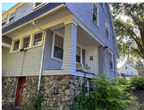
Figure 2: Lack of guards at basement, rear stair, and exterior porch
