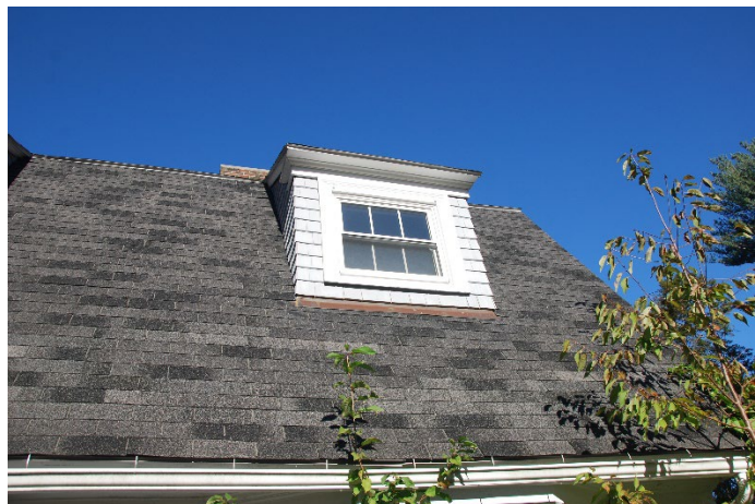
Gutter above entry soffit could be causing water damage at soffit
