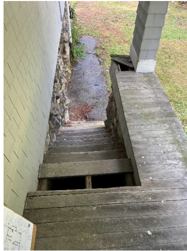
Figure 4: Missing treads and decking at rear stair
