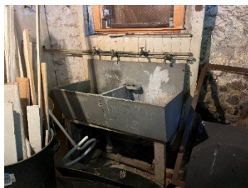
Basement Laundry Tub
