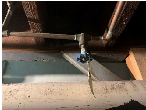
Main Water Service
