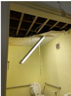
Ceiling at 1 st floor lavatory
