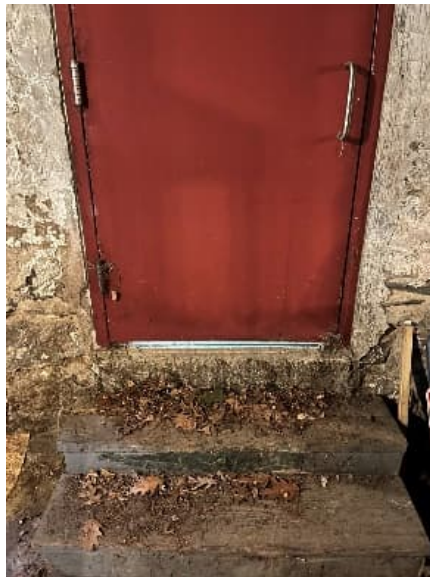
Figure 8: Non-compliant landing on inside of door
