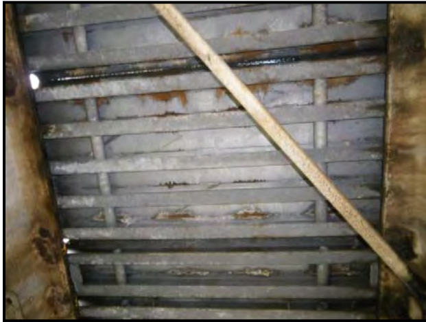
Figure 2-13 Typical Deck Panel Condition
