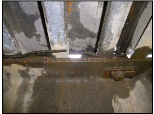
Figure 2-14 Loose Deck Connection, Broken Neoprene
