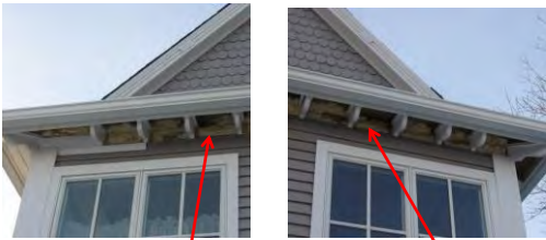
Holes in framing and missing foam sealant discovered in soffits
