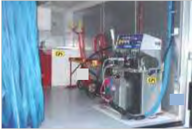
Mobile Spray Rig (Bulk foam)
