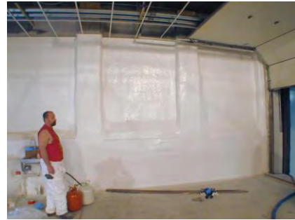
Bituminous VB coating loses bond due to heat-of-reaction
