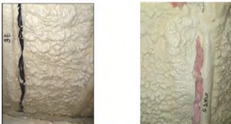
Pictures of cracks along rafters in the House attics. The one on the right has been temporarily stuffed with batt insulation until the remediation work begins.
