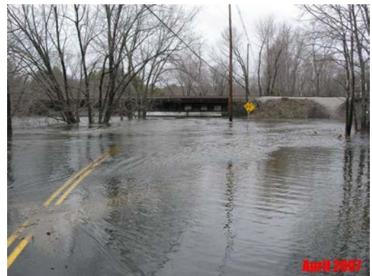
Figure 2: Flooding of MacPherson Road on April 18, 2007
