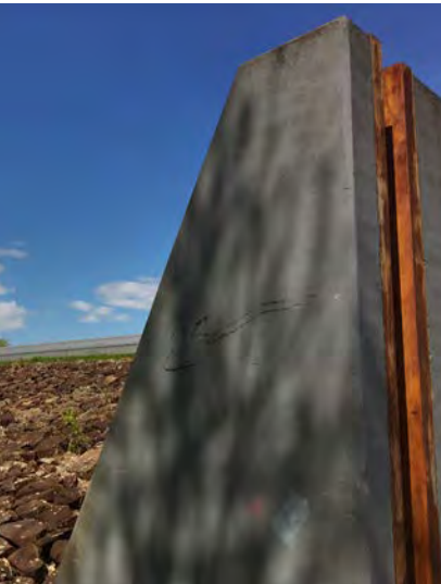
The earth dike and concrete flood wall along the Mill River, which can be considered both a vulnerability and a strength for Northampton.
