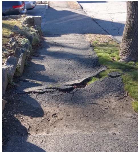
An asphalt sidewalk with root damage.
