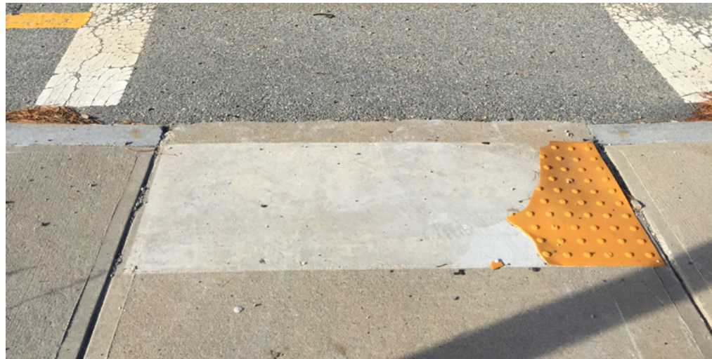
An example of a detectable warning panel in need of replacement.
