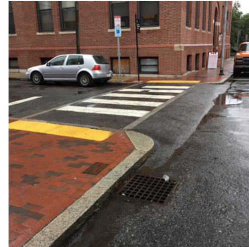
Figure 18. Raised crosswalks encourage yielding to pedestrians and reduce vehicle speeds.
