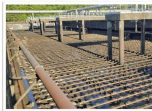
Aeration nozzles in the secondary treatment basin at the SRWTF
