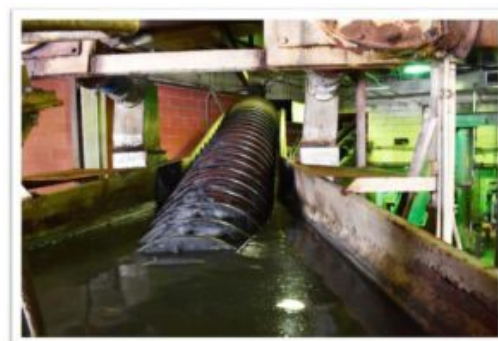
Existing grit cyclone in the SRWTF
