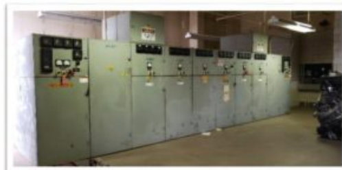
A 1970s era electrical panel in the SRWTF
