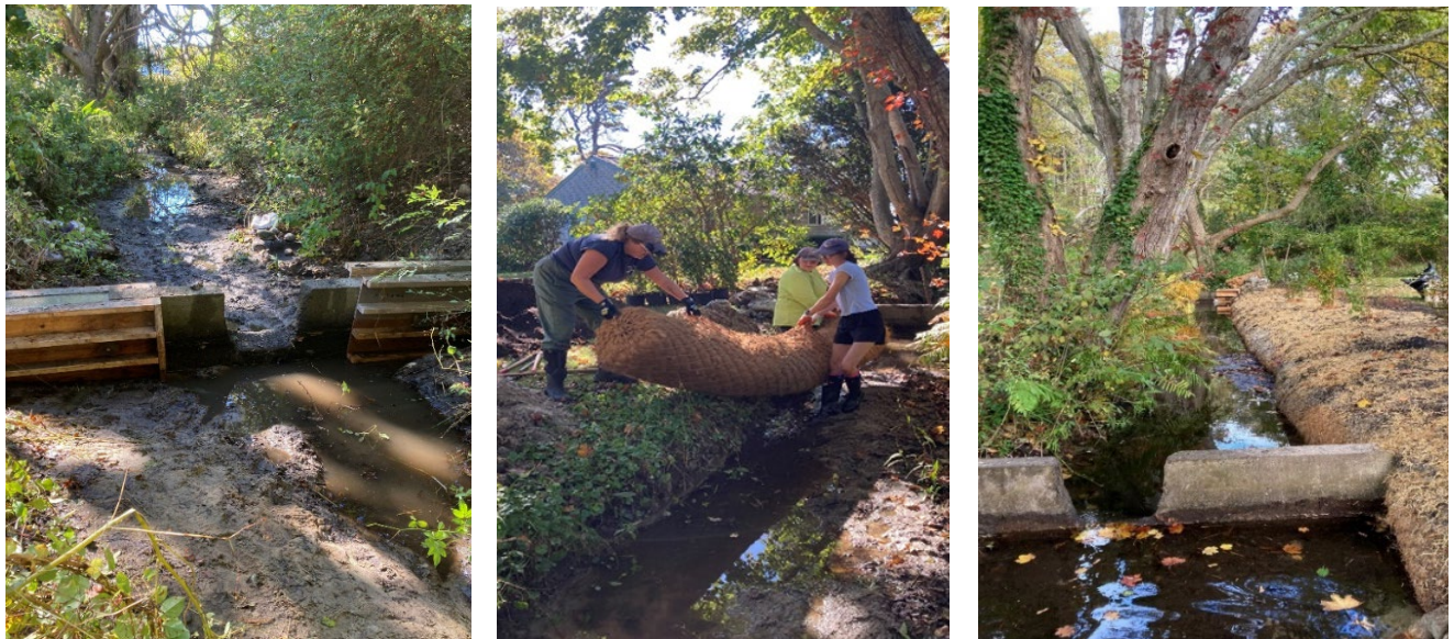
Figure 49. Repair to concrete fishway weir at Stillwater Pond, Chatham (left), fiber roll installation (middle), and final site appearance.
