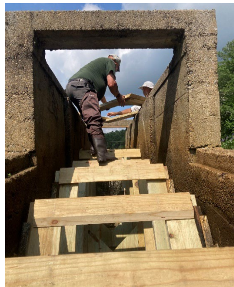
Figure 46. DMF Fishway Crew replacing Denil baffles at Elm Street Dam on the Indian Head River, Pembroke/Hanover.
