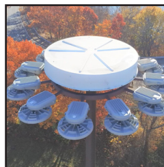
high mast lighting
