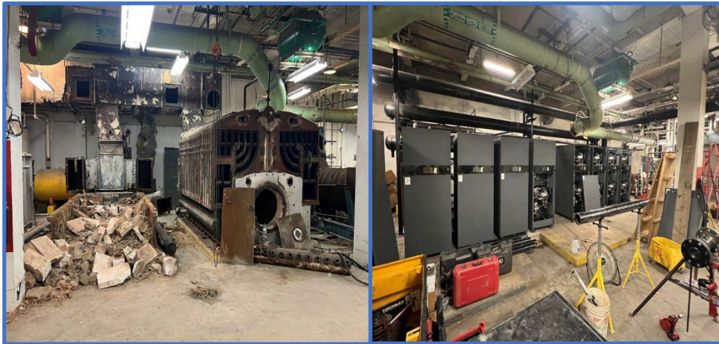
BOILER UPGRADE BEFORE AND AFTER- DELCASTLE VO-TECH. OLD BOILER(LEFT): TWO 10-MILLION BTU BOILERS. NEW BOILER (RIGHT): EIGHT 2-MILLION BTU HIGH-EFFICIENCY BOILERS.
