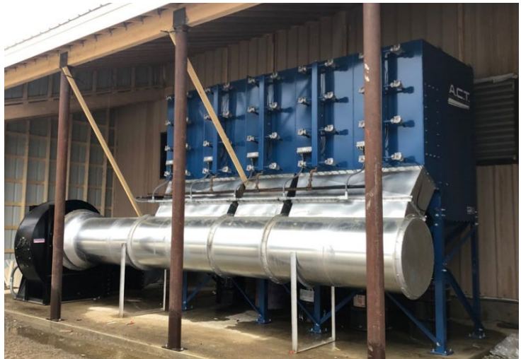
HIGH-EFFICIENCY DUST COLLECTION SYSTEM AT THE ROBBINS LUMBER FACILITY IN NORTH SEARSMONT, MAINE.
