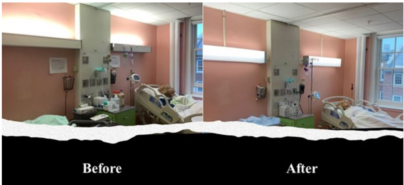
IMAGES OF THE OLD (LEFT) AND UPGRADED (RIGHT) LIGHTING AT THE ELENOR SLATER HOSPITAL
