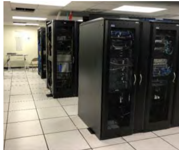
Post-investment 10 Park Plaza Server Room
