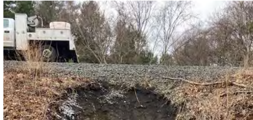
Culvert failure on the Knowledge Corridor in Northampton, MA
