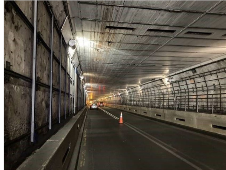
Sumner Tunnel before restoration
