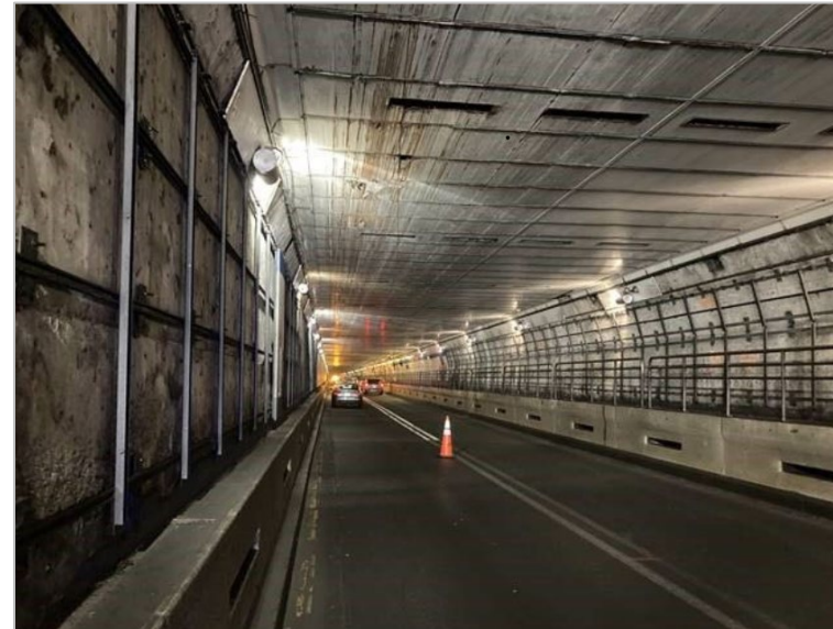
Sumner Tunnel before restoration
