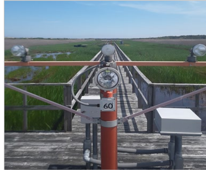
Provincetown approach lighting system
