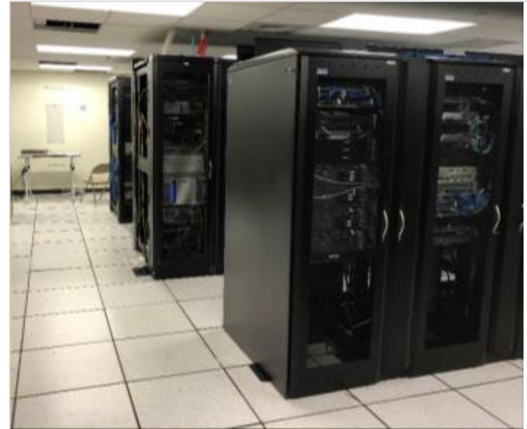
State Transportation Building server room after investments
