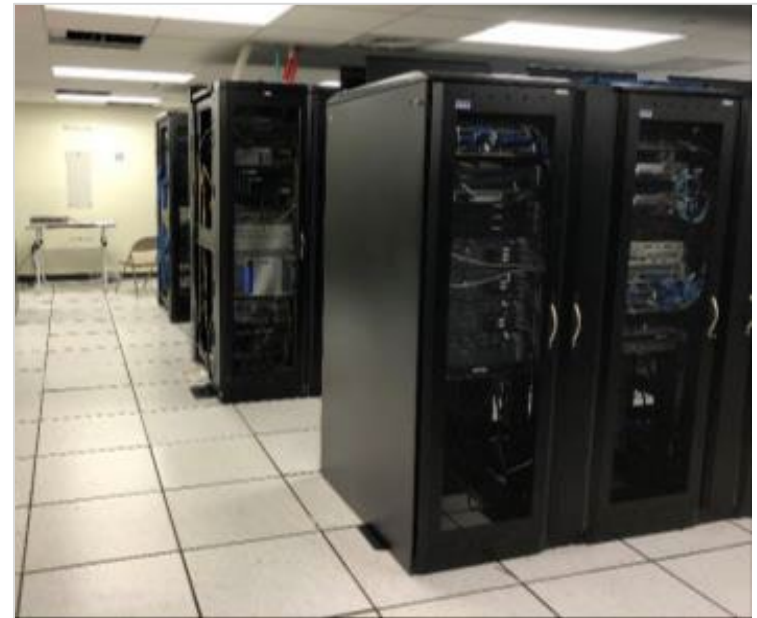
State Transportation Building server room after investments
