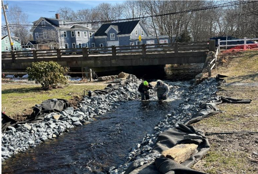
Figure 43. DMF staff monitoring water velocity in bypass channel for Veteran's Park fish passage improvements on the South River, Marshfield.
