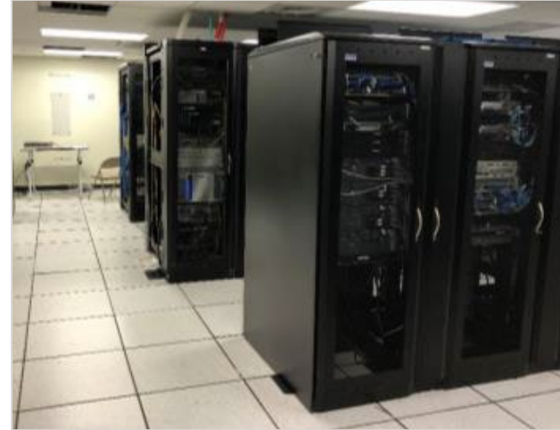
State Transportation Building server room investment
