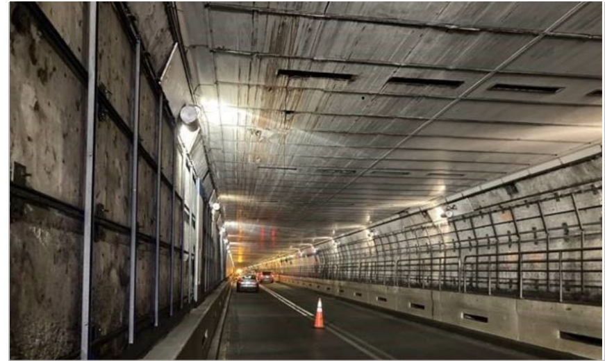
Sumner Tunnel before restoration
