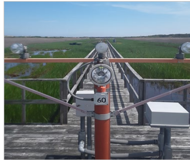
Provincetown approach lighting system
