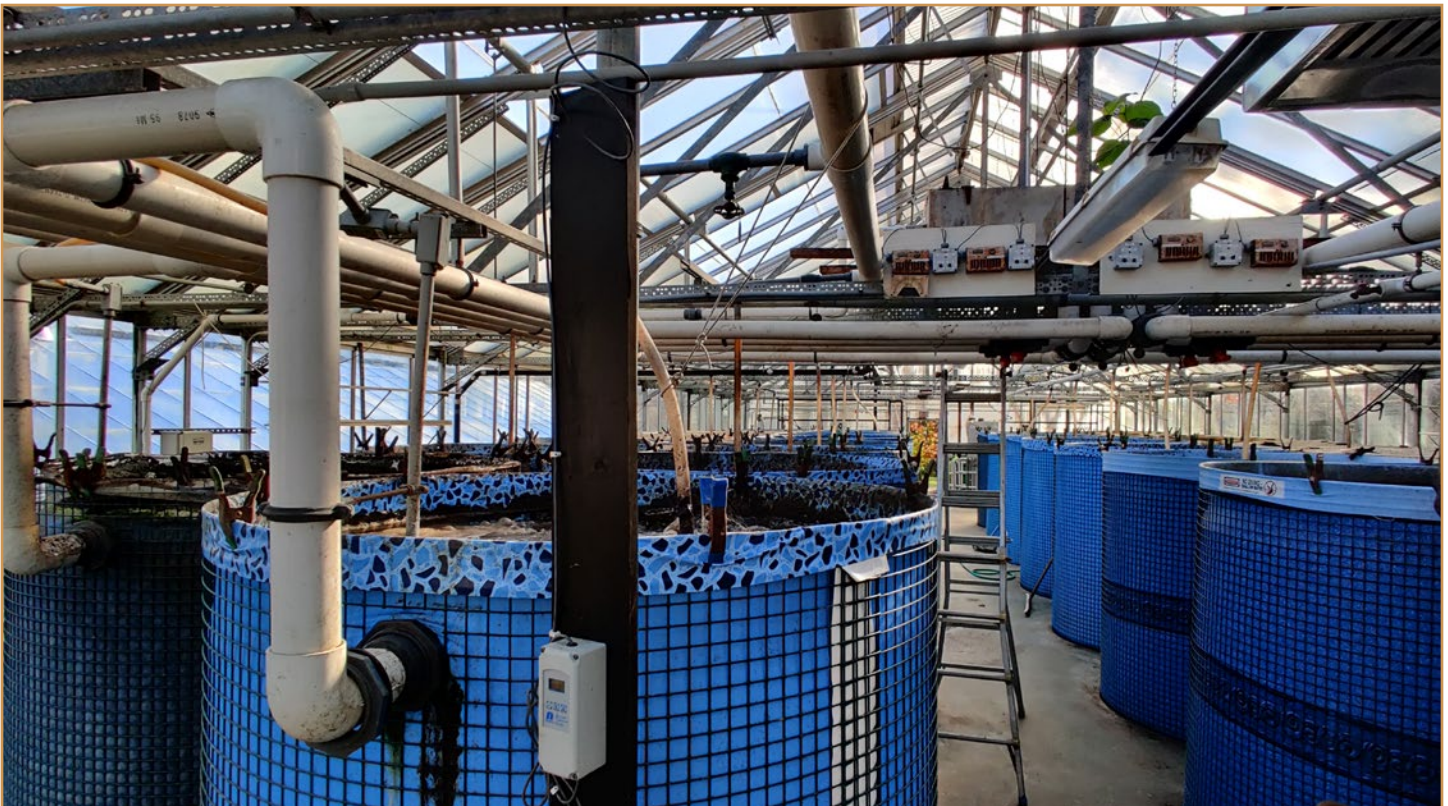
A small-scale water treatment system in Ashfield.
