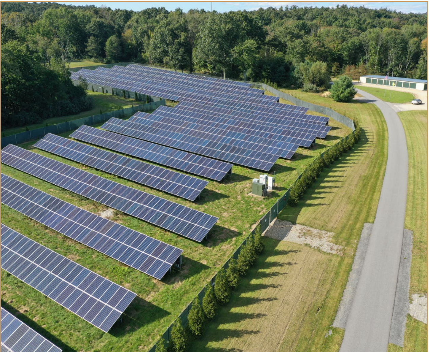
A solar array in Spencer.
