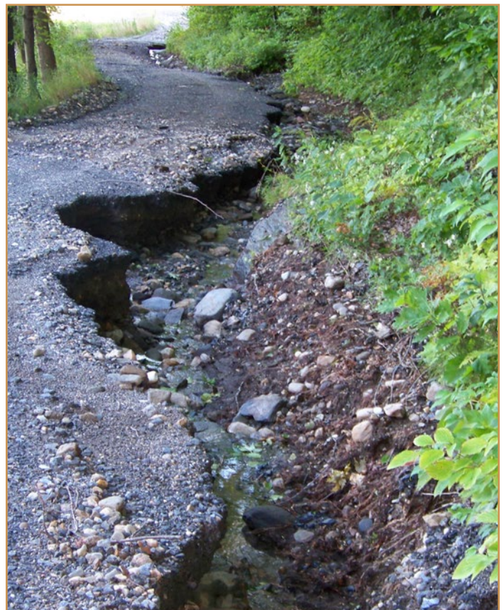
A washed-out unpaved road in Ashfield.
