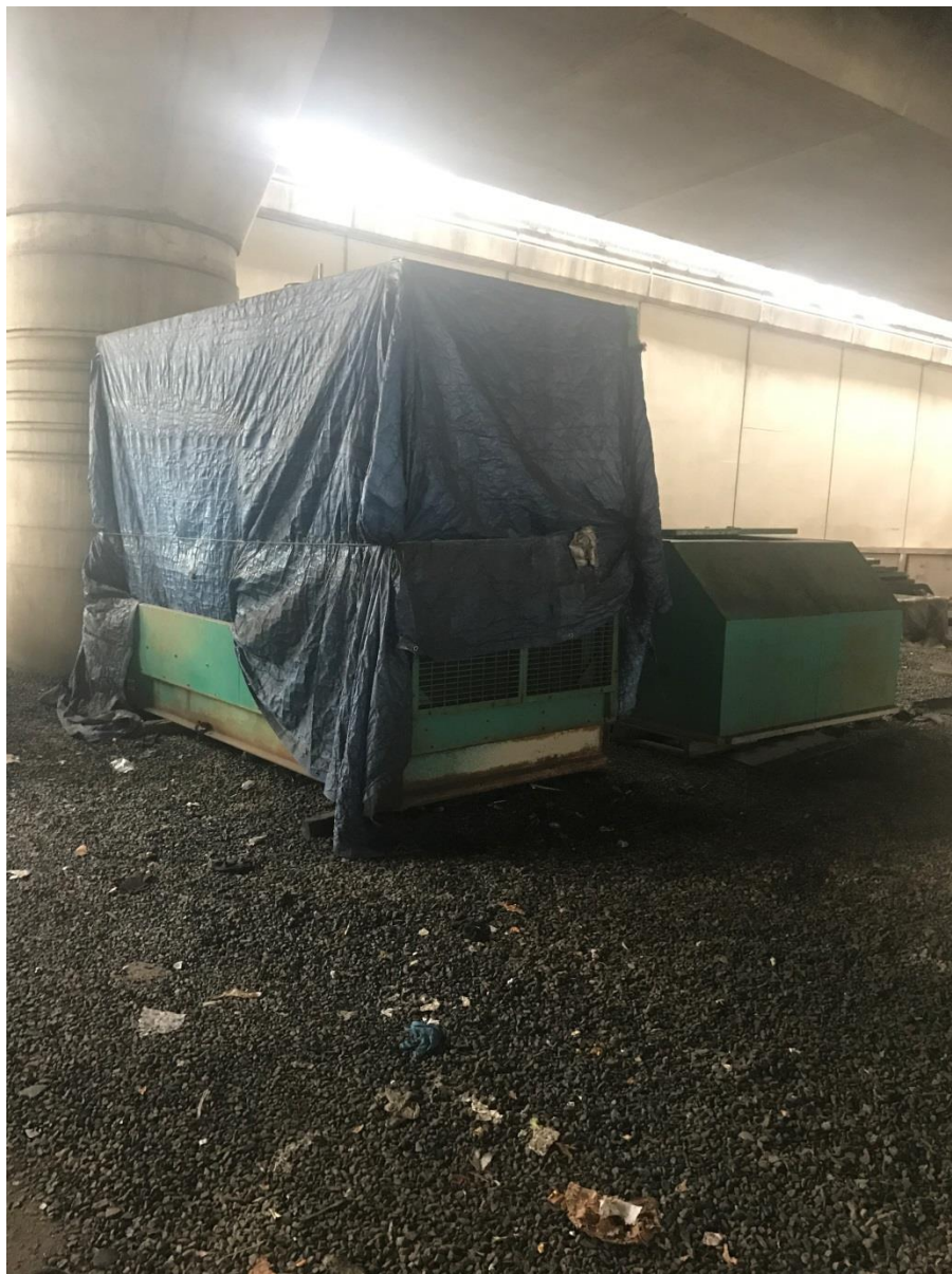
ISAU photo of one of the natural gas generators that MassDOT paid for, but never used. MassDOT houses this generator behind the District Six Headquarters building on Kneeland Street in Boston, underneath Interstate 93. This photo was taken on November 2, 2017.
