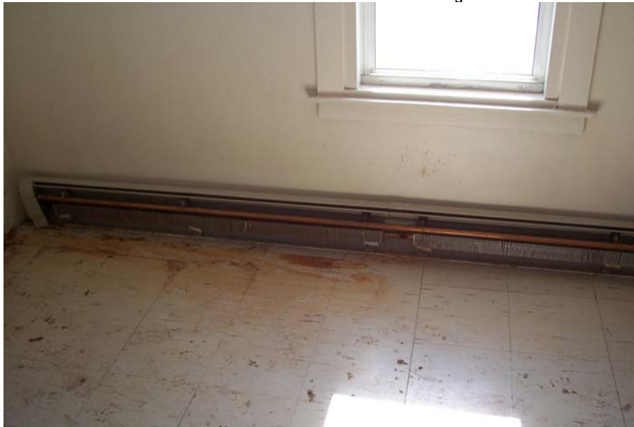
Unit 5D Baseboard Heat Cover Missing
