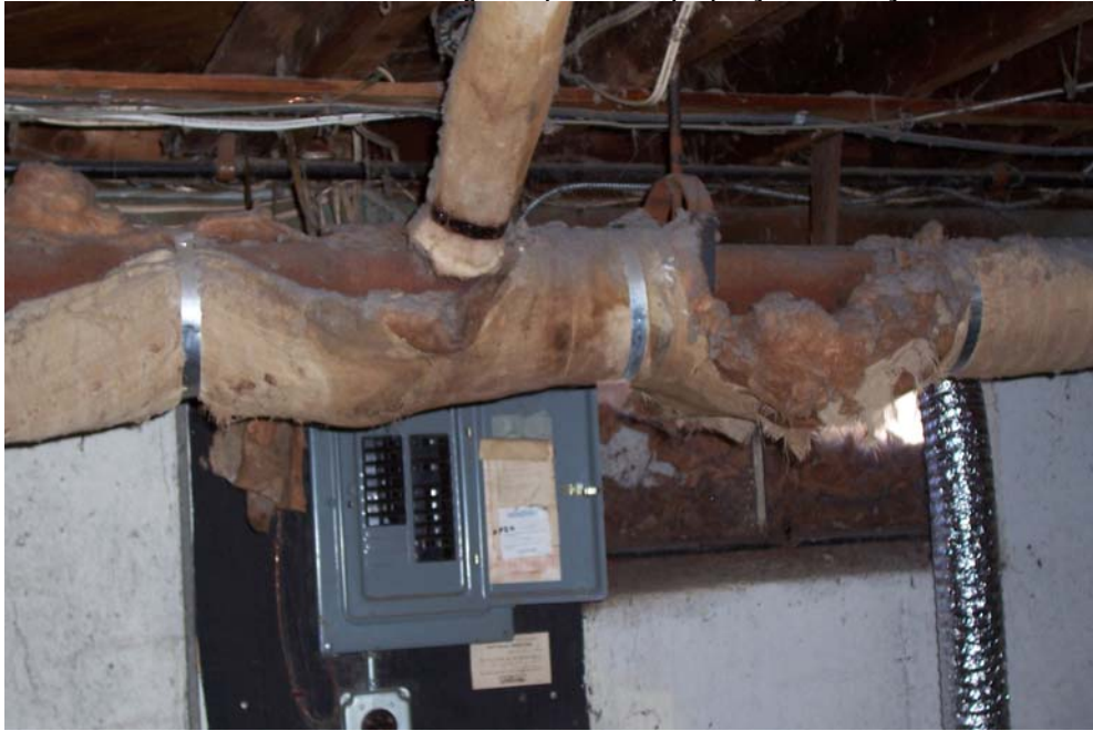
Unit 2D Insulation Coming off Pipes and Improperly Vented Dryer
