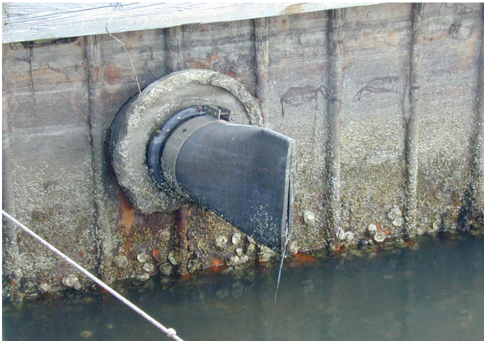
Figure 10. Flapper valve located at the end of discharge of the STS units at the Wychmere Harbor site.
