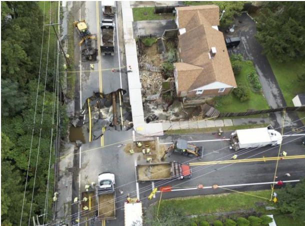
MassLive, September 2023: Erosion caused by flooding at culverted Reservoir Brook in Leominster September 11th & 12th, 2023 in Minority & Low-Income EJ block group.. As much as 11" of rain fell in Leominster during the event. No flood zone is mapped around Reservoir Brook.
