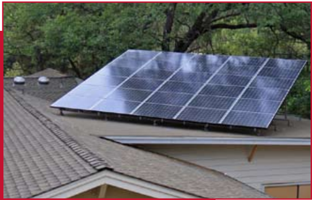
Photovoltaic arrays installed on the roof of a home. Photo by Velo Steve.
