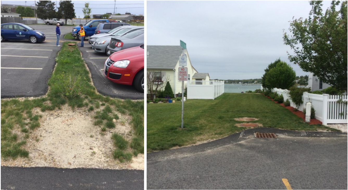
Figure 5.14. Existing Conditions in Parking Lot, Site 32A (top) and Beach Access Way Site 32B (bottom)
