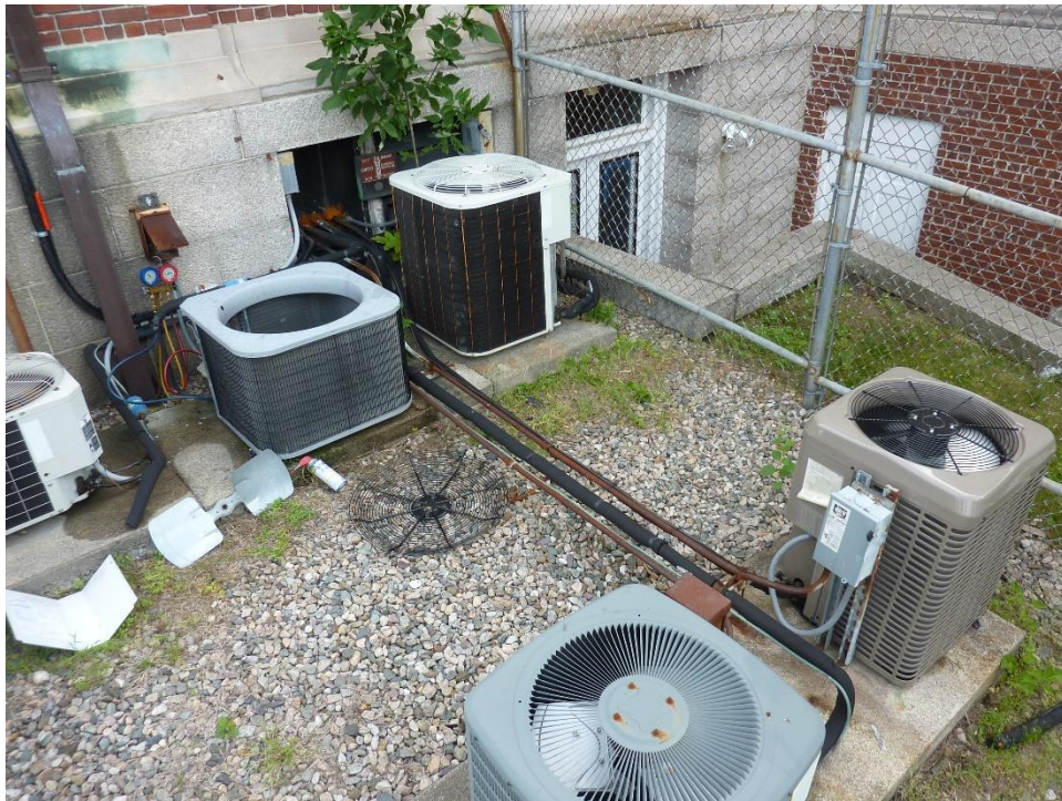
Photo 4 – Outdoor Condensing Units
