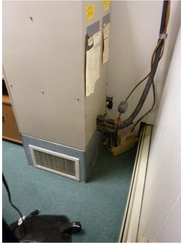
Photo 1 –Representative Split-System Air Handler
