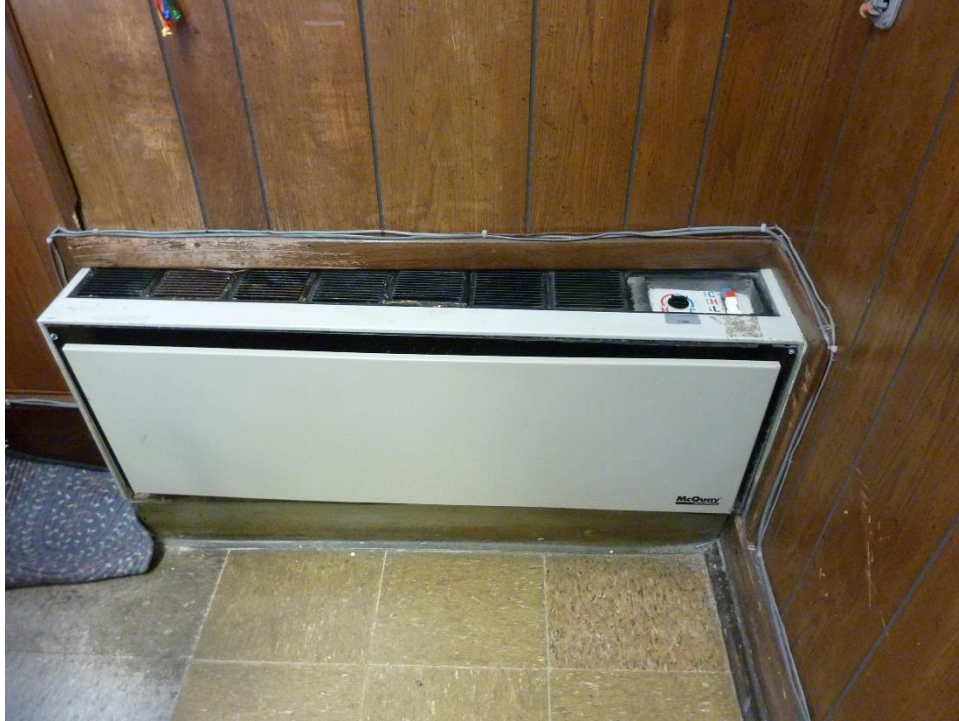
Photo 3 –Representative PTAC Fan Coil
