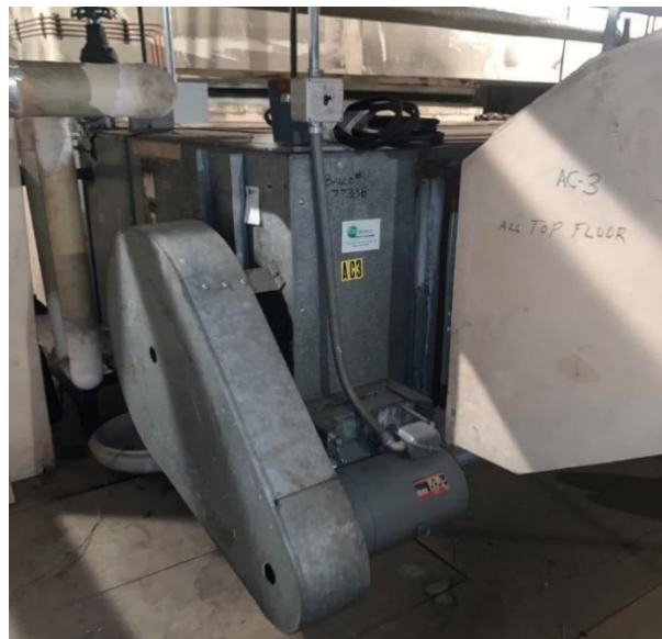
Photo 1 – Typical Air Handler
