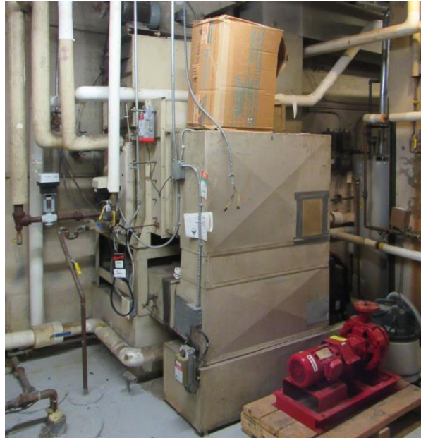
Photo 2 – Air handler AHU-1
