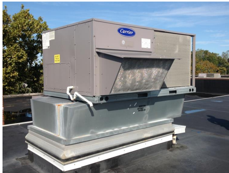
Photo 1 – Representative Rooftop Air Handler
