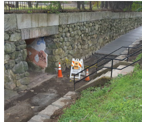
New walkway and drainage improvements near the Belmont Center Commuter Rail on Concord Ave. Photo credit: Town of Belmont, 2018, via Twitter.
