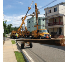
Photo: Routine pole and transformer replacement on Beech Street. Photo by Belmont Light, 2018, via Twitter.
