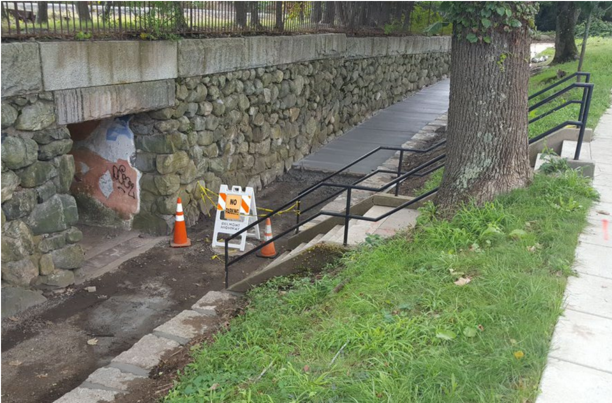
New walkway and drainage improvements near the Belmont Center Commuter Rail on Concord Ave. Photo credit: Town of Belmont, 2018, via Twitter.
