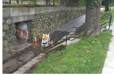
New walkway and drainage improvements near the Belmont Center Commuter Rail on Concord Ave. Photo credit: Town of Belmont, 2018, via Twitter.
