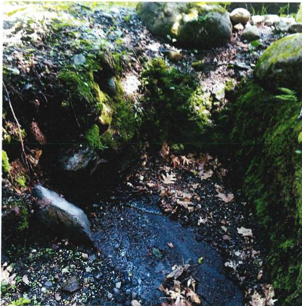
Photo 2: Culvert Inlet with Limited Capacity
