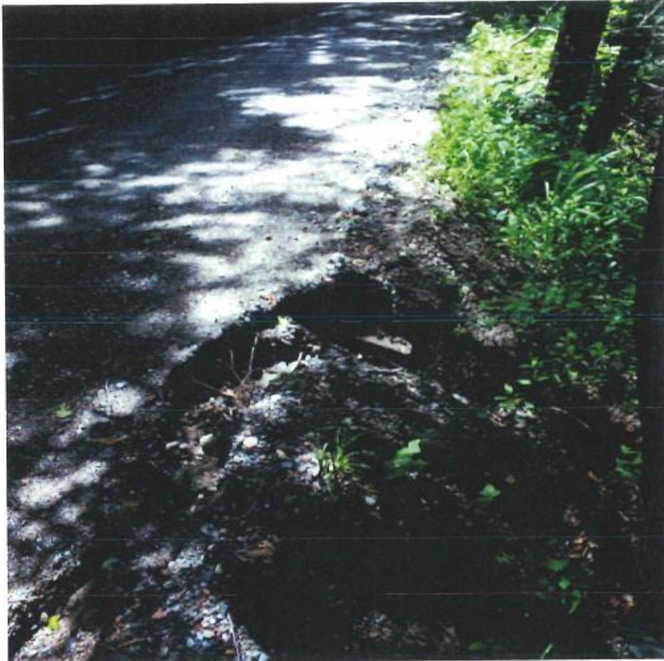
Photo 3: Eroded Side Slope on Downhill side of Road at Haigis Branch Road
