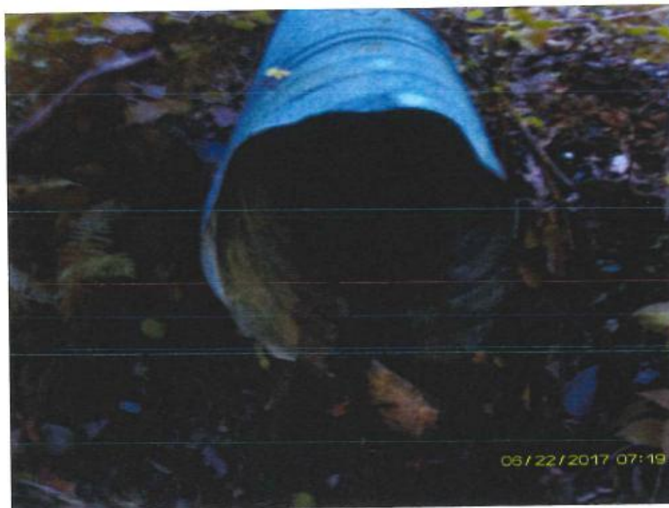
Photo 1: Corroded Metal Culvert at Outlet
