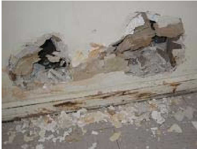
705 Family Housing Development 115 Boardman Street, Apt. #2, Bedroom #2 Walls are Damaged, Covered with Health-Endangering Mold, Floor is Worn and in Disrepair
