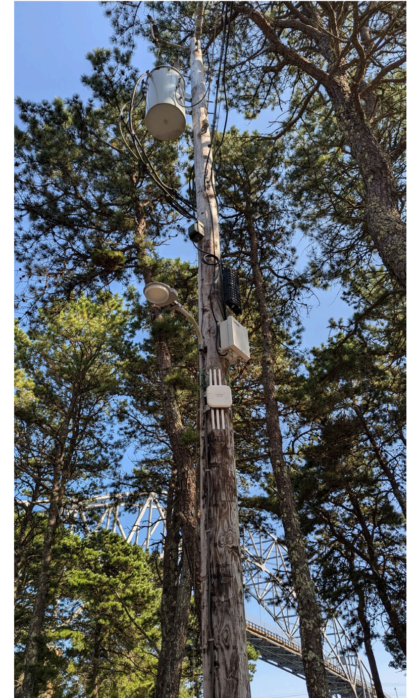
Existing Wi-Fi infrastructure
