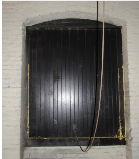
Photo 2 – Sealed outdoor air opening.
