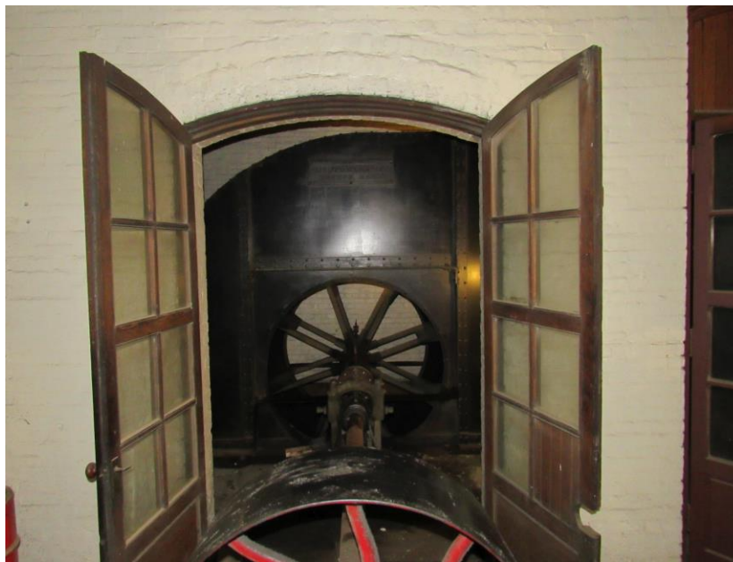
Photo 1 – Blower Seen Through Return Air Doors
