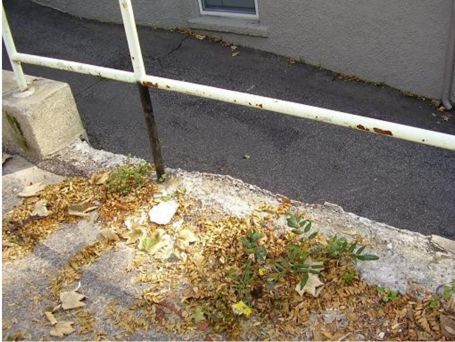
667-1 Development – Chipped/Broken Concrete Stairway Colonel Floyd, Marion Street
