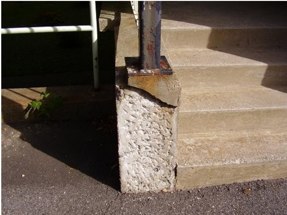
667-1 Development– Chipped/Broken Concrete Stairway Colonel Floyd, Foster Street
