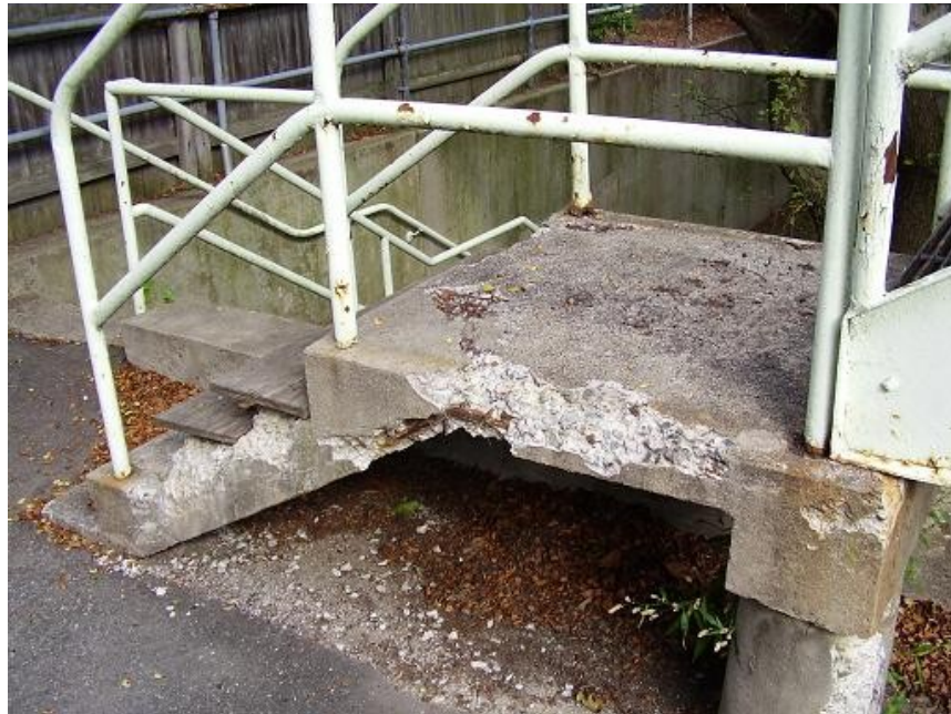
667-1 Development – Deteriorating Concrete Stairs and Rails Colonel Floyd, Foster Street
