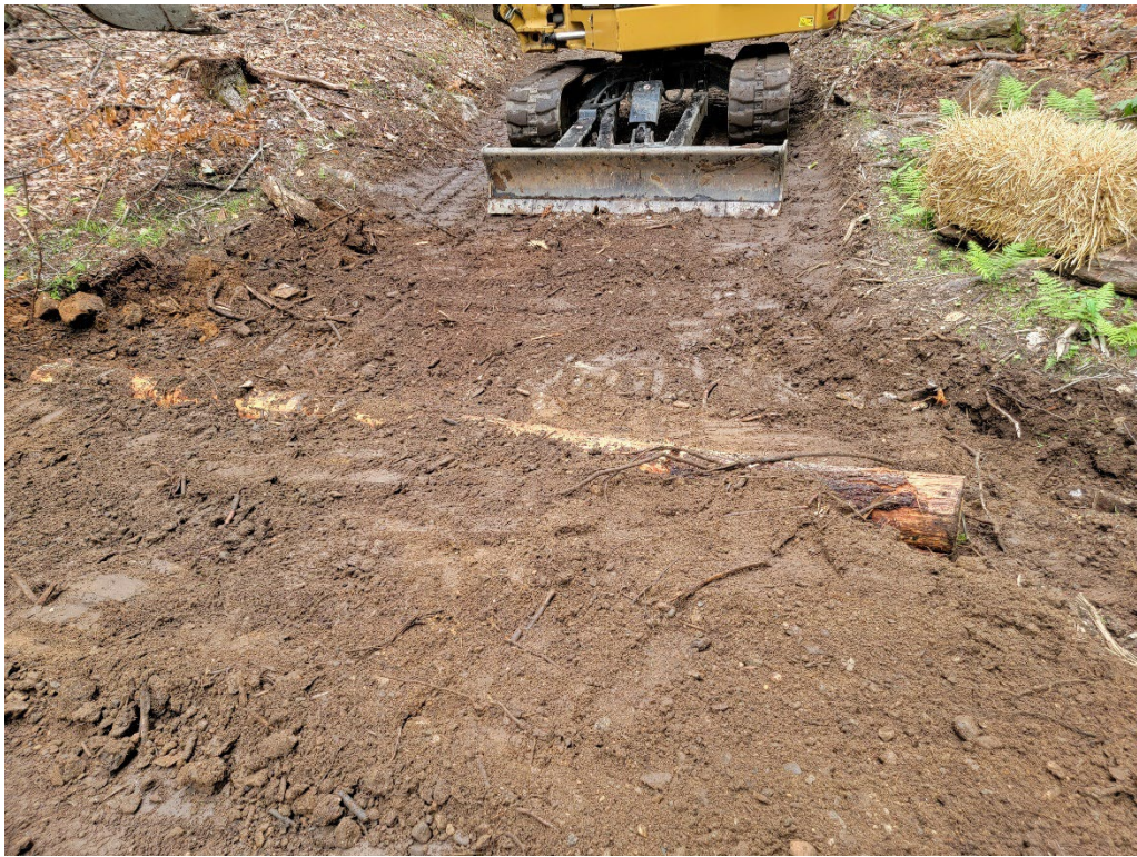
Installation process of a log reinforced water bar on the active harvest. C-SIP 5 Demo day, Town of Athol. Photo credit: Sara Wisner
