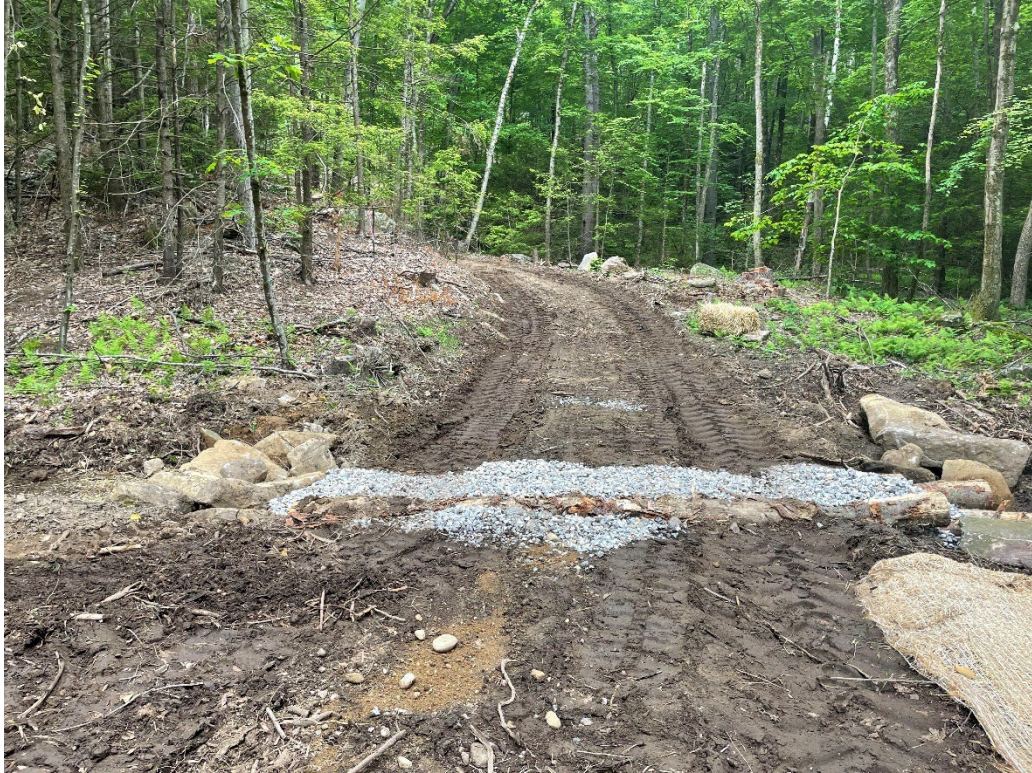
Finished Installation of a log reinforced water bar on the active harvest. C-SIP 5 Demo day, Town of Athol. Photo credit: Michael Downey
