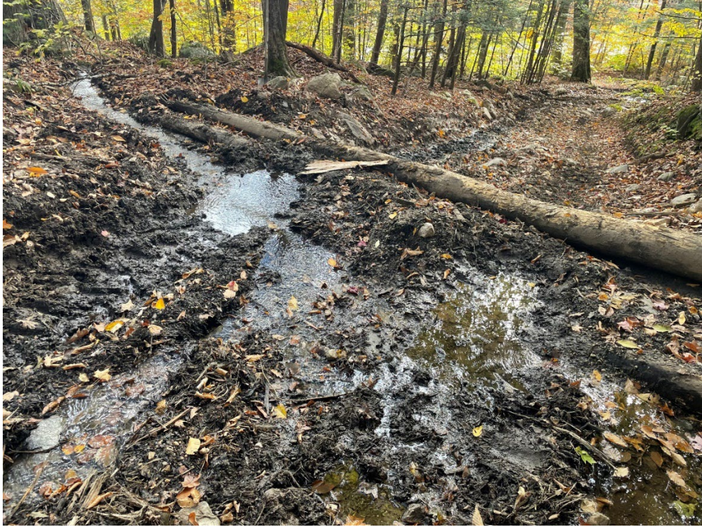
Example of log reinforced water bar on the active harvest. Photo credit: Colin Mettey
