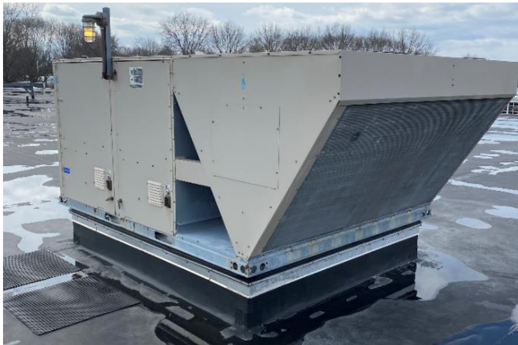
Photo 1 – Representative Air Handler
