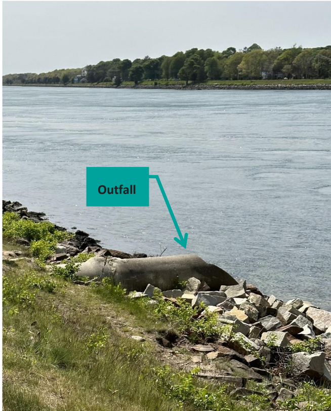
Exhibit 4.10-6. 24-Inch Pipe Outfall at Cape Cod Canal (Bourne South Quadrant)
