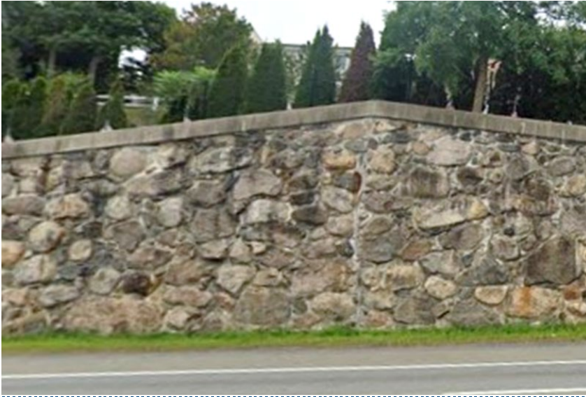
Exhibit 8-8. Example of High Exposure MassDOT Stone Masonry Wall
