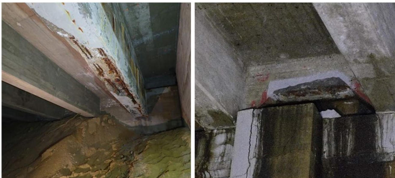
Exhibit 2-3. Concrete T-Beam Deterioration (Bourne Bridge)
