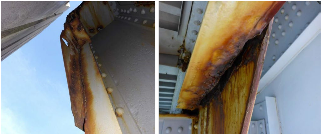
Exhibit 2-1. Truss Joint Gusset Plate Deterioration (Sagamore Bridge)
