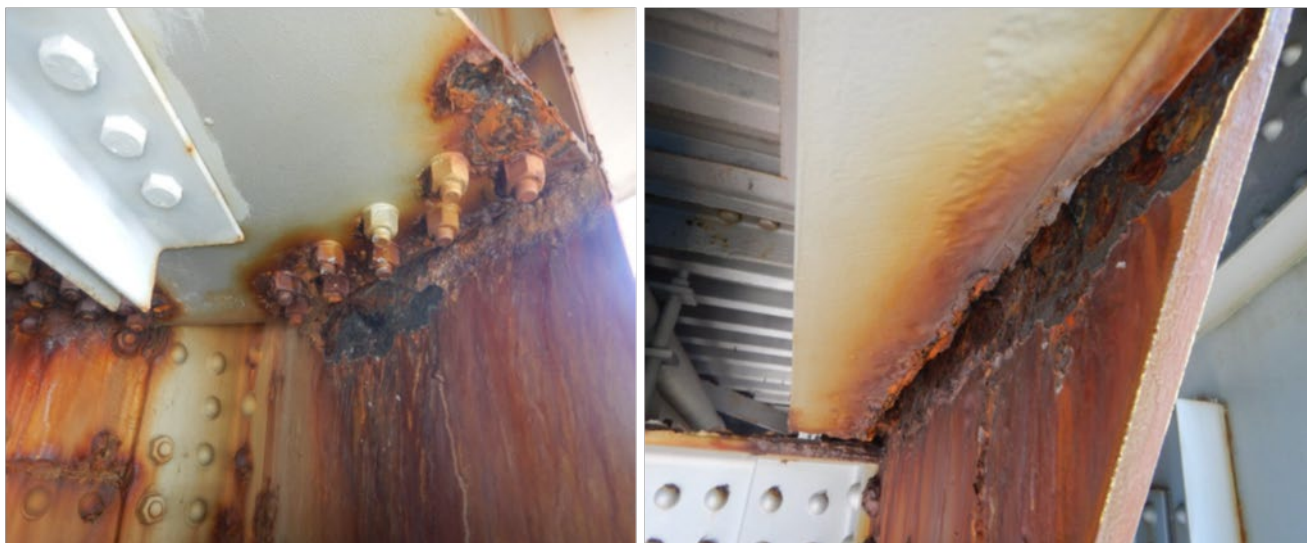
Exhibit 2-2. Truss Joint Gusset Plate Deterioration (Bourne Bridge)
