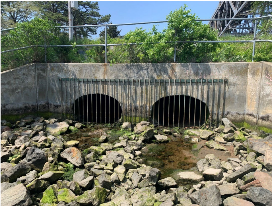
Exhibit 4.10-5. Twin 43-inch by 68-inch Elliptical Pipe Outfalls (Bourne North Quadrant)
