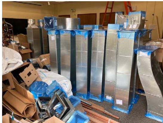
Ductwork in conference room ready for installation
