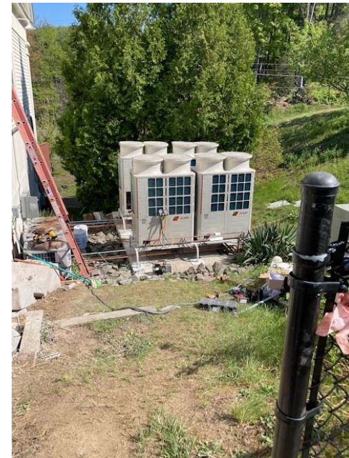
Outdoor VRF condensers
