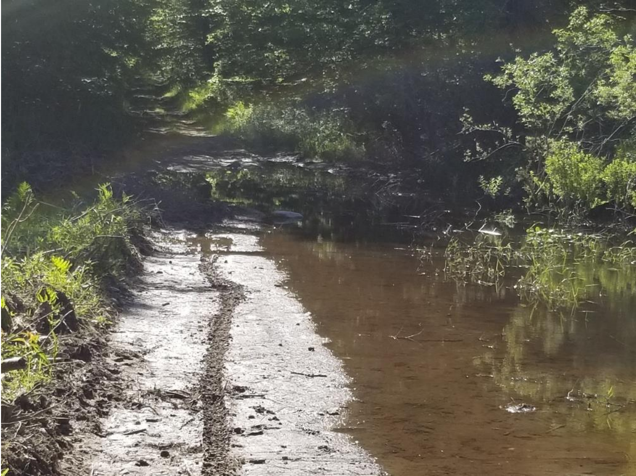
Partially Flooded Segment of Dodd Road, Town of Sandisfield
