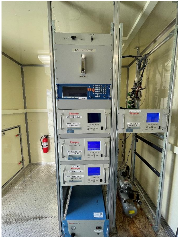
Figure 3-4: CO-NO-NO 2 DST Monitors Enclosure
