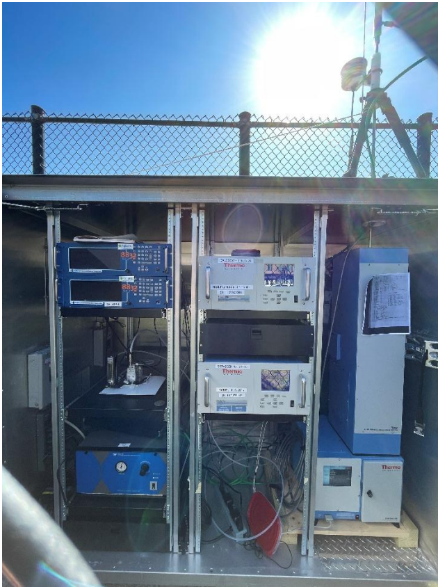
Figure 3-3: CO and PM 2.5 Monitors in Equipment Shelters
