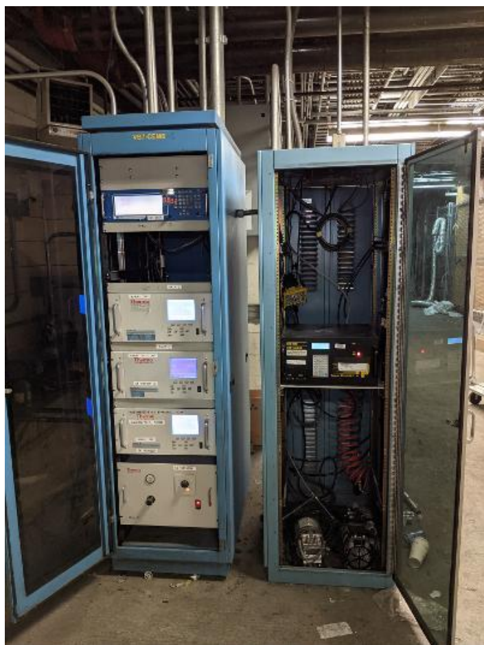
Figure 3-2: CO and PM 2.5 Monitoring Units at VB 7 Exhaust
