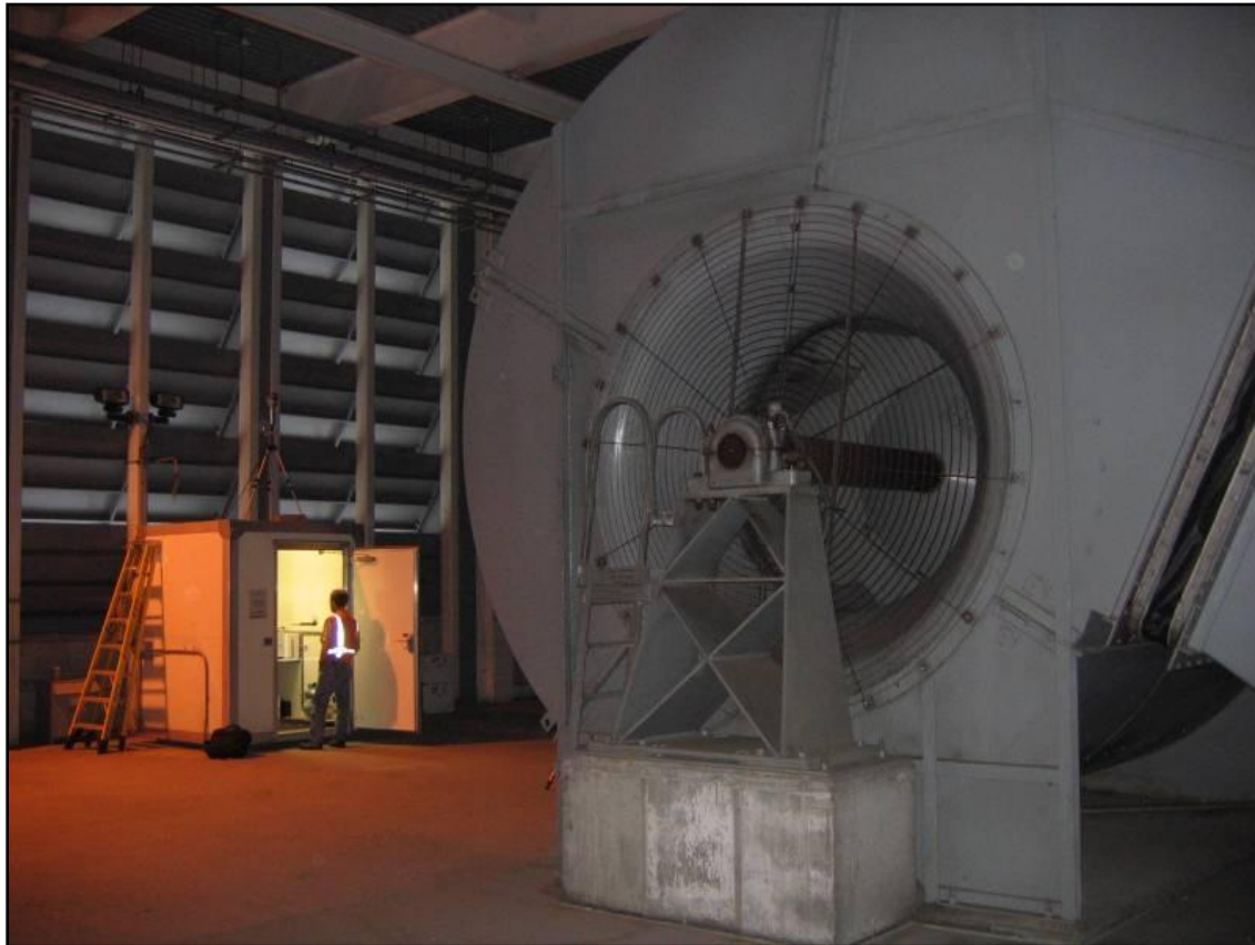
Figure 1-15: Supply Fan at VB 7 Air Intake Floor
