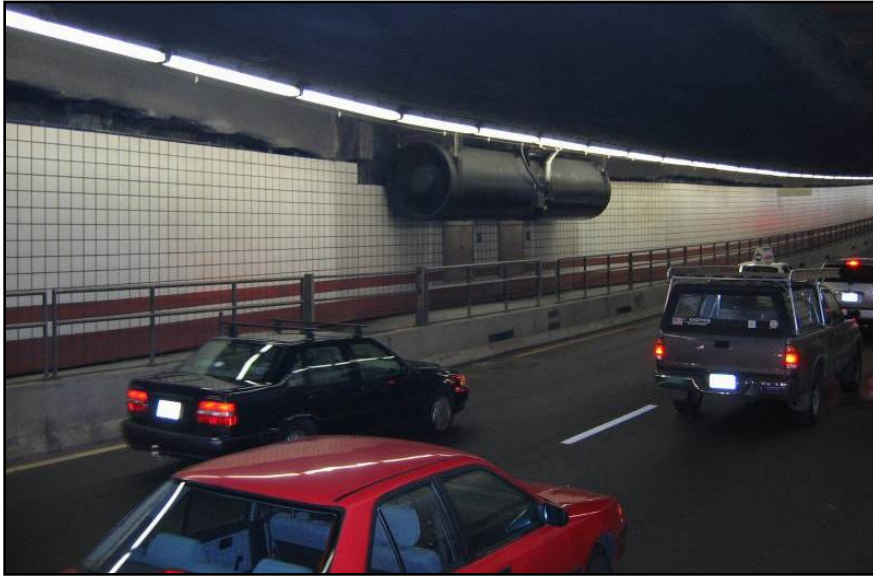
Figure 1-16: Jet Fan at Longitudinally Ventilated Ramp
