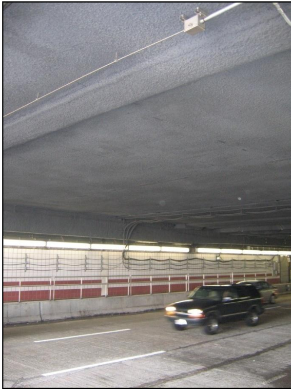
Figure 3-1: CO Ceiling Monitoring Probe at DST
