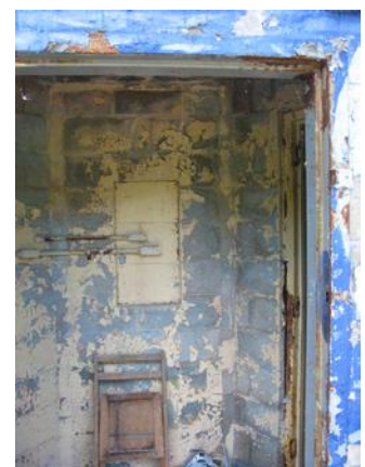
Interior and exterior water damage at the Martini Shell
