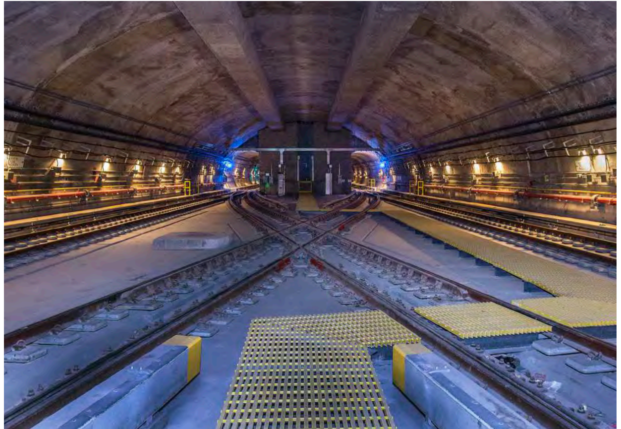
Tunnel for the 7 Line Extension in New York to the 34th Street / Hudson Yards Station
